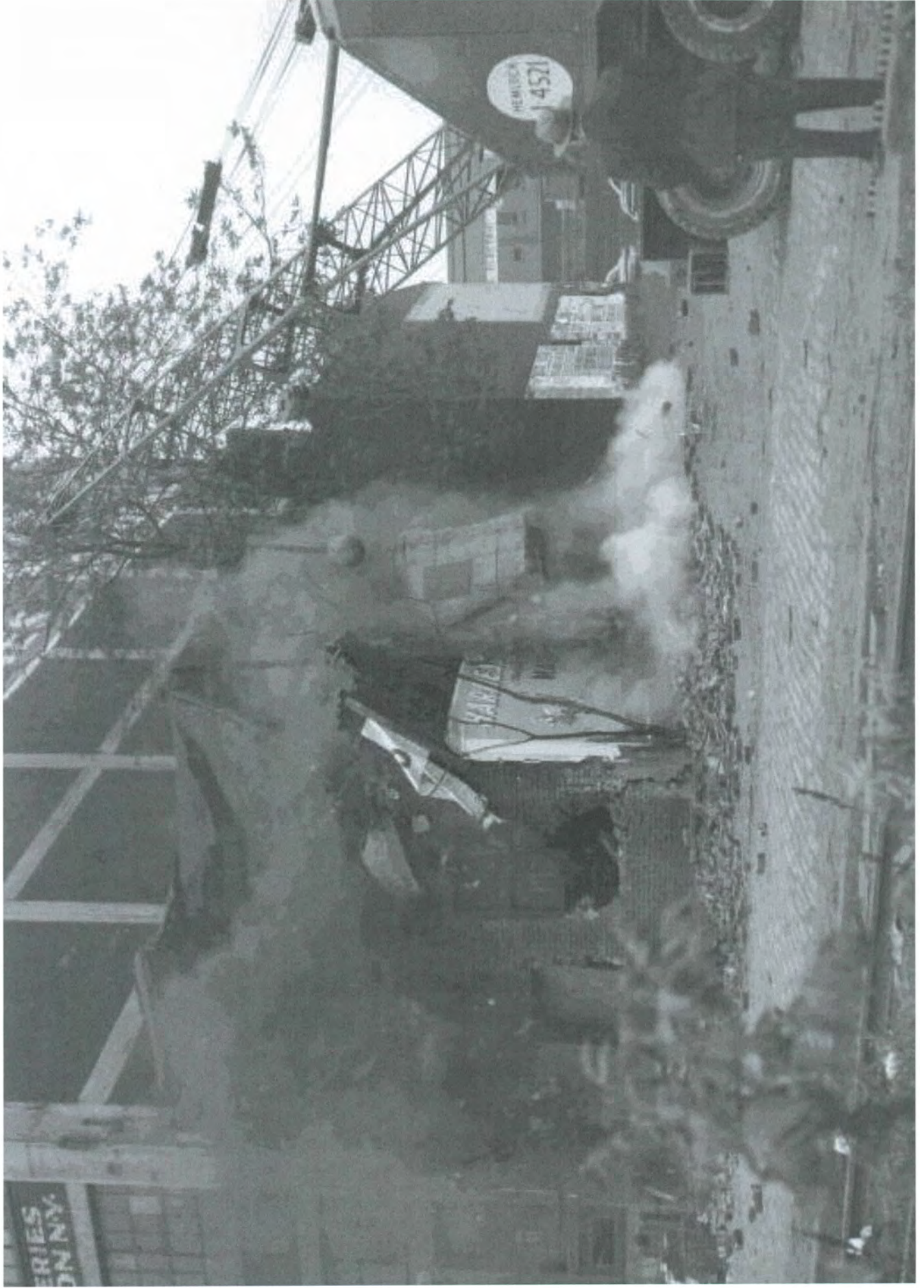
Image 3.4: Commencement of Demolition for the Point Park and Gateway Center Project, May 18, 1950 Source: University of Pittsburgh Digital Archives: Historical Society of Western Pennsylvania
